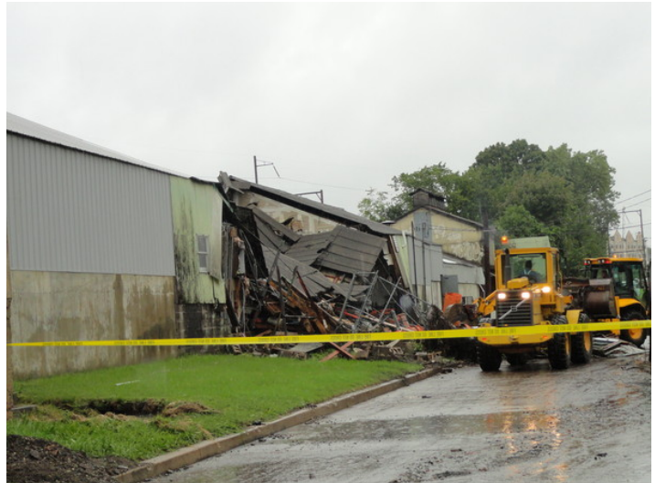
Figure 1.7 Damage to warehouse and West Maple Street after Tropical Storm Lee in 2011.
